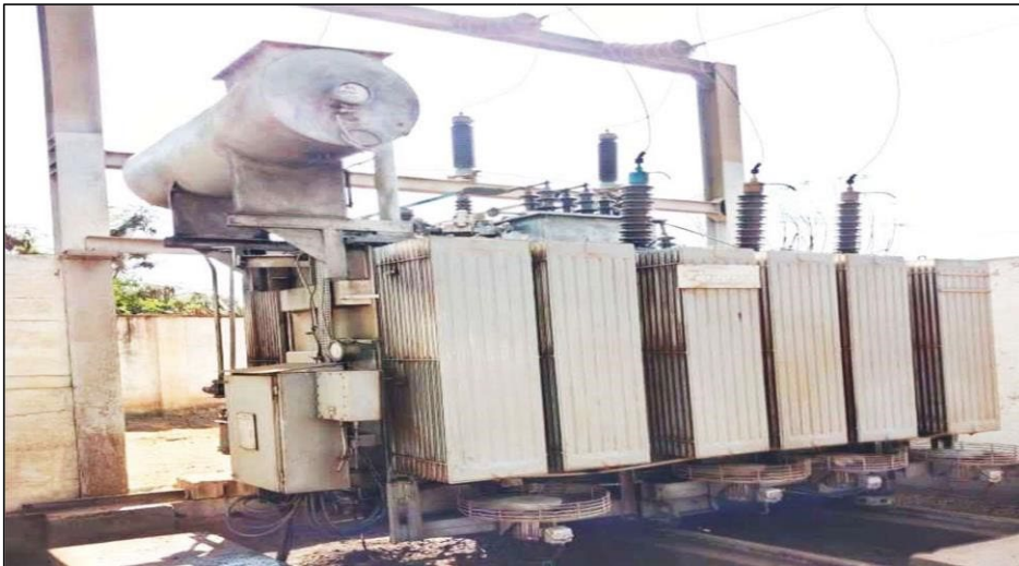
Figure 3. Unilu substation power transformer
